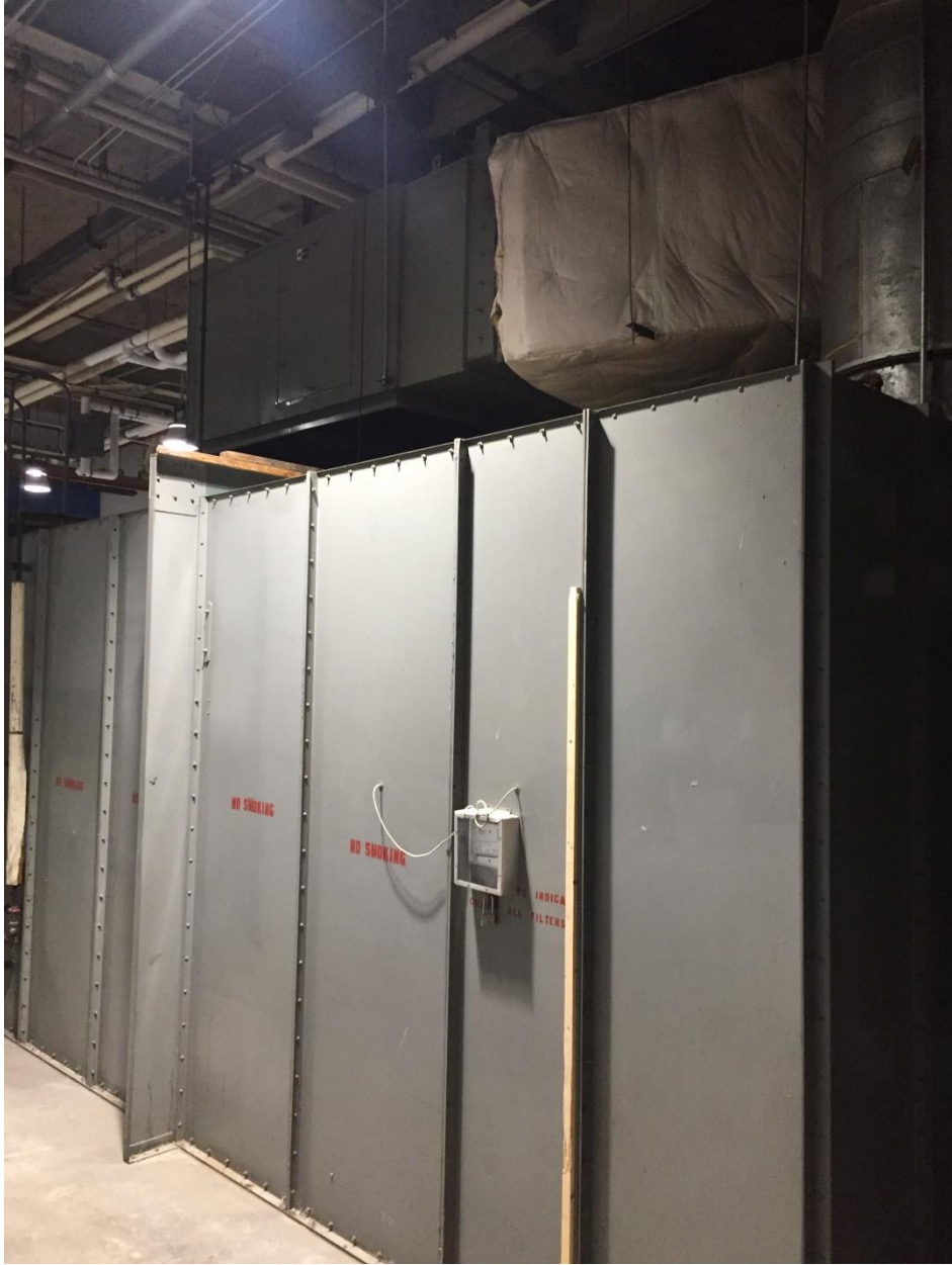
MAU Unit above paint booth
